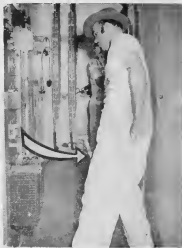
First step in the cutover was Adolph Arends pulling the main fuse (see arrow); this "killed" the old exchange for the first time since it was installed about 1934.
